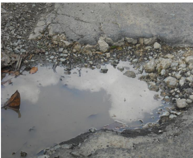
Sumber : Abdul Hamid (2016) Foto 4: Lack of binding to the lower course (Potholes & Slippage), Kab. Sintang
